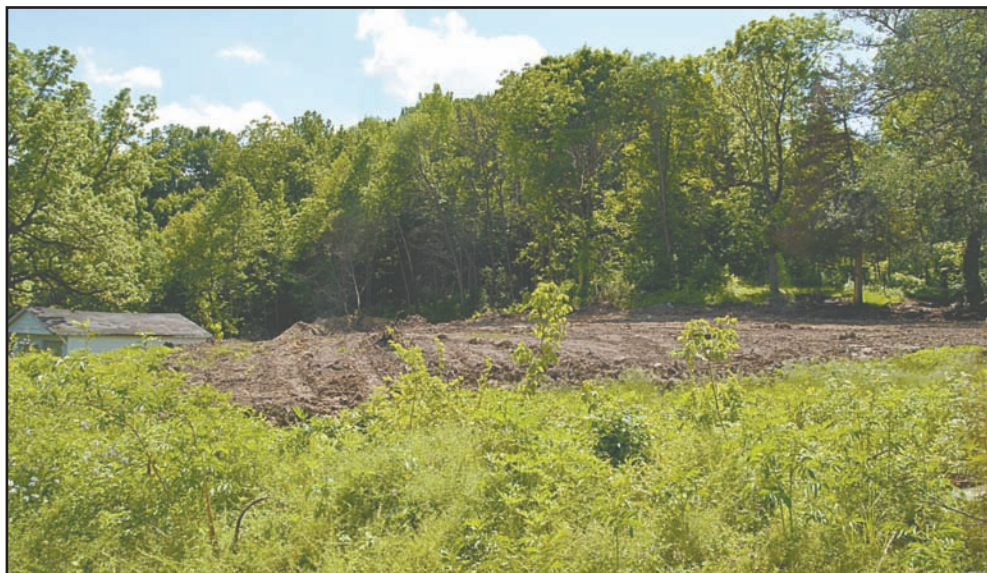
Jeremy Mueller purchased this land to the north of his property and demolished a number of old buildings. He hopes to see a house built on this property in the future. (Chris DeBack photo)
